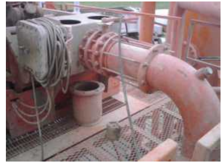
Figure 10 Inlet Pipe & Flange Connected to Header Box
