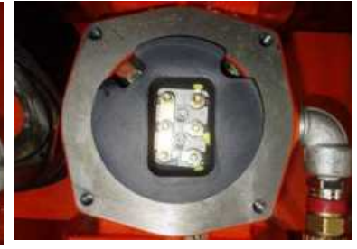
Figure 27 Thick Isolator - Motor Leads Not Showing
