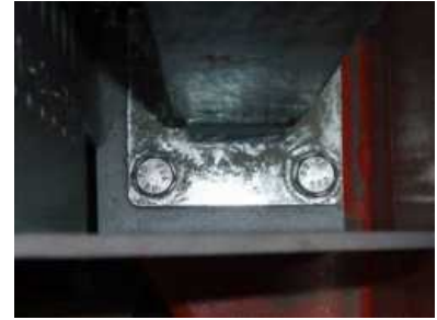
Figure 39 Overhead View of Hardware Base
